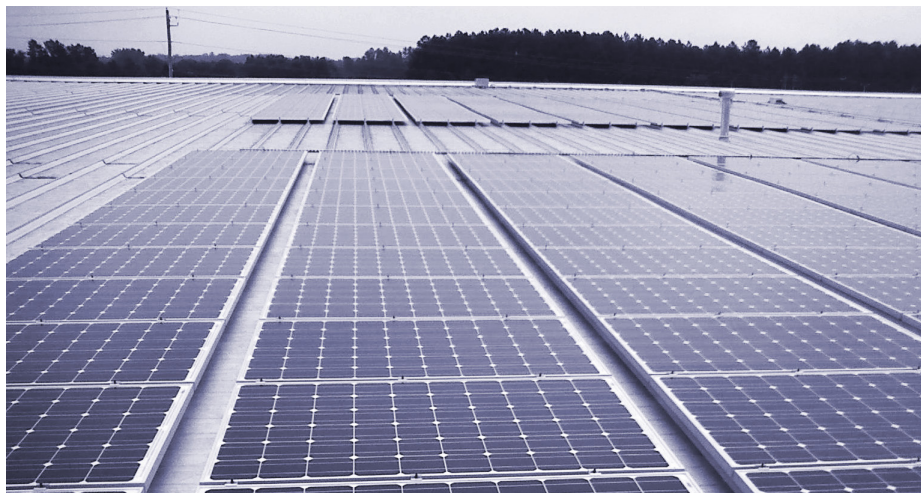
Other Green Power EMC Solar Facility
